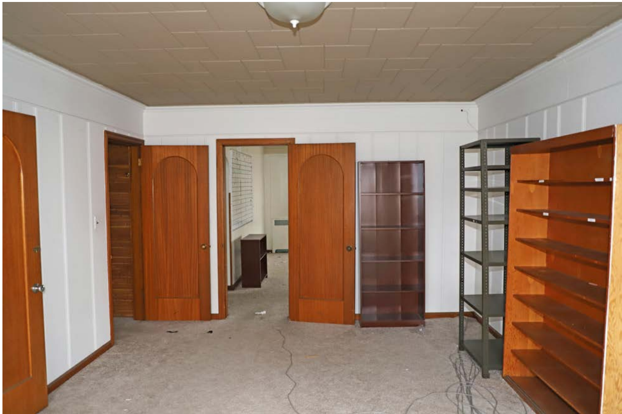
Photo 37. Second floor, bedroom, central, looking east. The center doorway opens to the living area.
